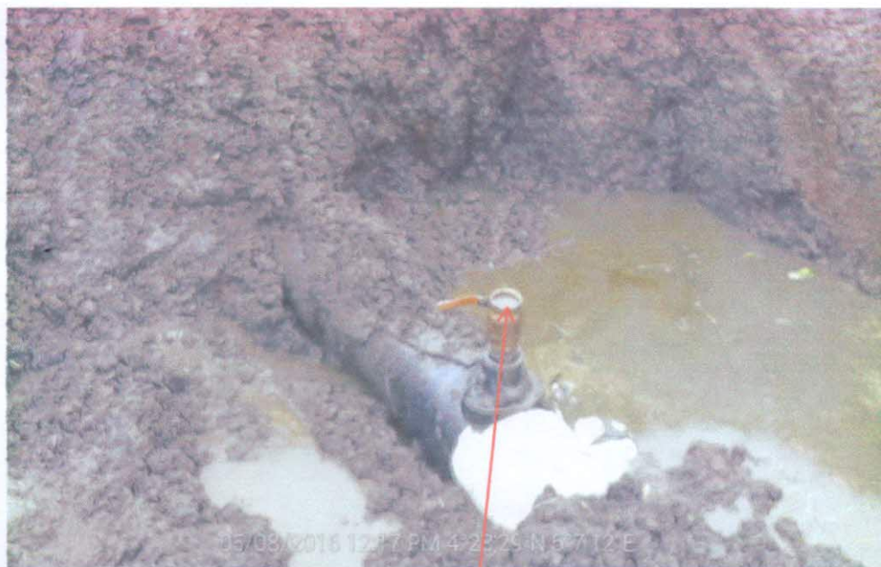
NON-LEAK POINT (4INCHES VALVE) INSTALLED
